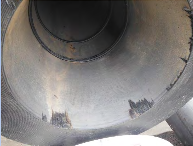
HDPE Wear at Flange
