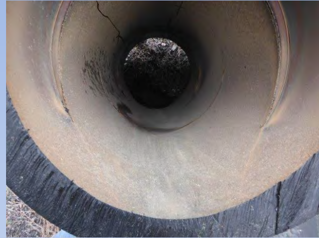
HDPE Wear at Bottom
