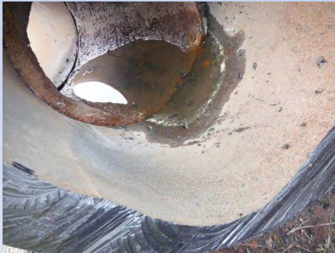
HDPE Wear Downstream from Turn
